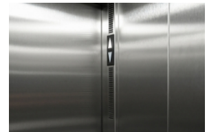
Signalisation Landing direction indicator in the door portal
