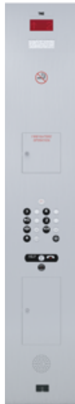
Car operating panel
